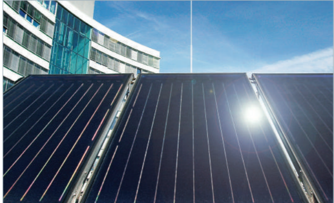
Solar power plants (collectors)
