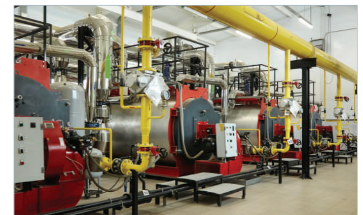
Large-scale heating systems
