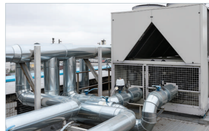
Building cooling systems
