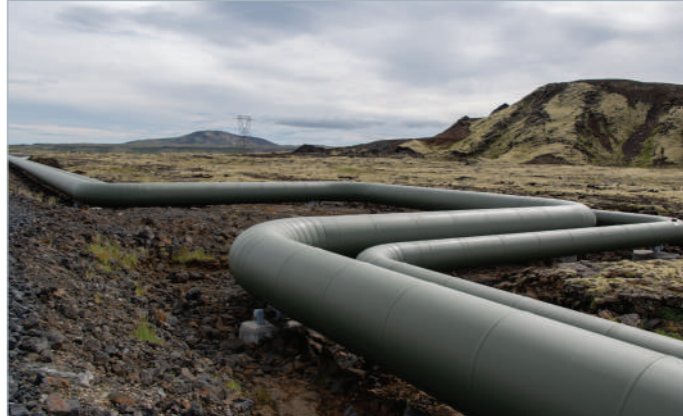
District heating supply
