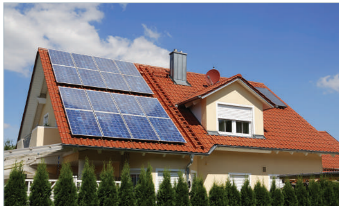
Solar heating systems (collectors)
